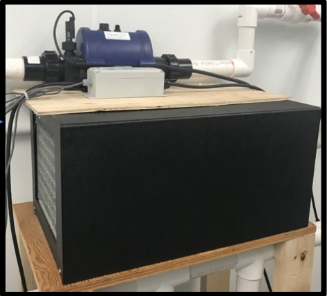
Heater and Chiller
